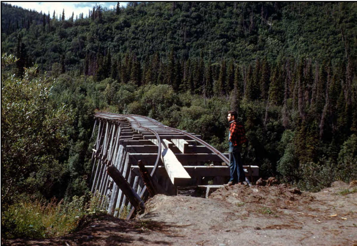
ARC crewmember Fred Morey looks over the remains of the Fox creek trestle. The rails from Chitina to Fox Creek had been removed by this time.
