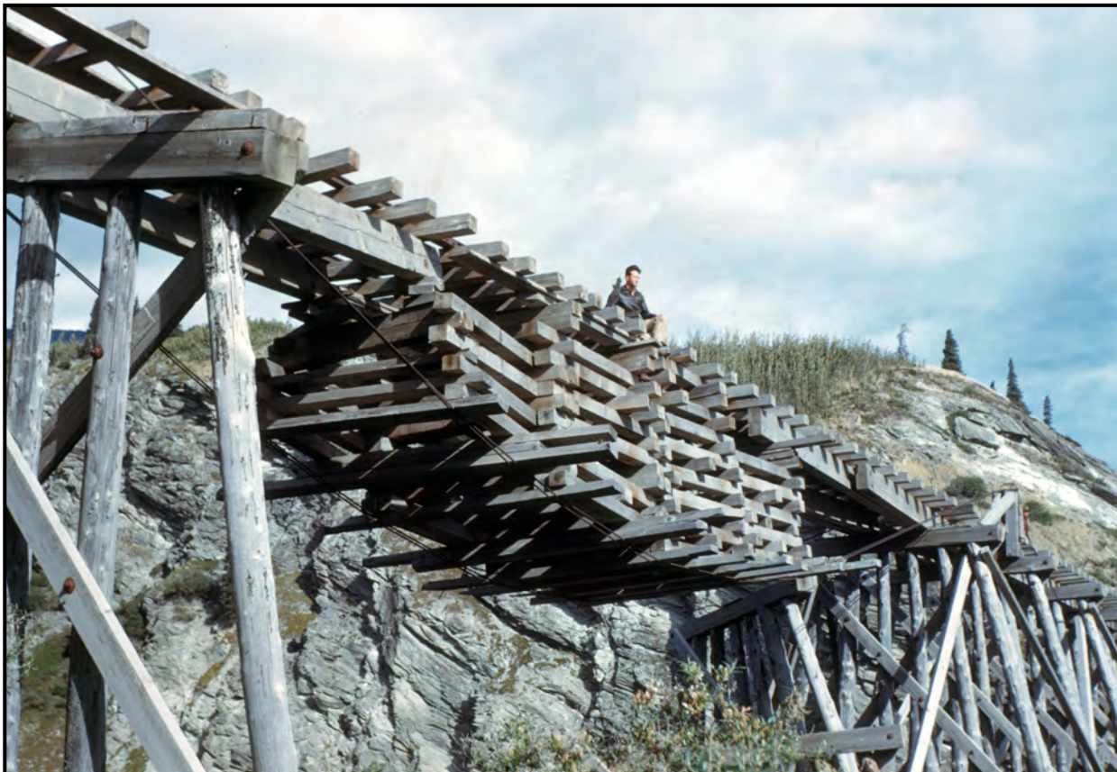
Bob Leitzell standing on the O'Brien Creek trestle. It is thought that O.A. Nelson had a hand in the ingenious suspension bridge type repair.
